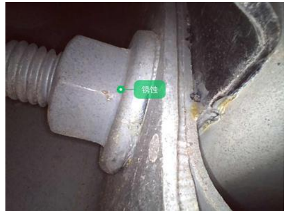
右前纵梁:锈蚀
